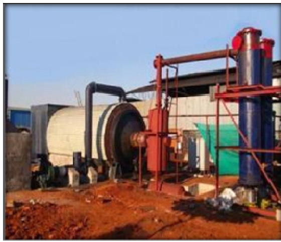
Figure 5 Plastic Pyrolysis Process Plant.
